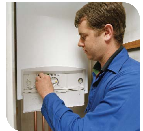
An example of a typical boiler
