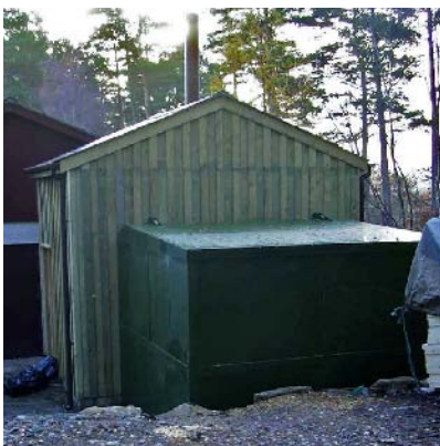
30kW (heat output) wood fuel system with the green hopper and boiler house attached to main building
