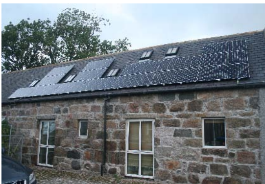
Pitch roof mounted, 3.60Kwp solar pv panels at Drumoak (image courtesy of AISSC Electrical and Solar)
