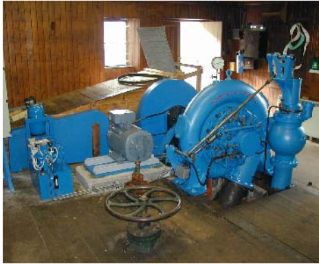
Gilbert Gilkes & Gordon turbine, courtesy of the British Hydropower Association
