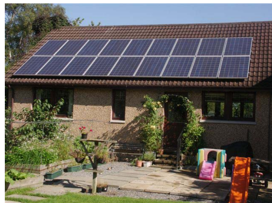
3.87 KWp pitch roof mounted solar pv panels of Aboyne (image courtesy of AISSC Electrical and Solar)
