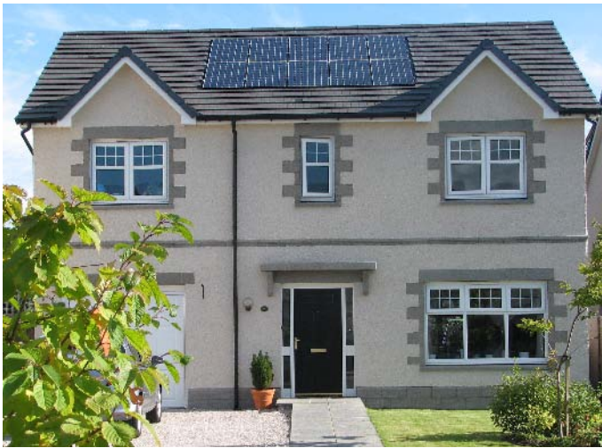
3.60KWp Pitch roof mounted solar pv panels of Aberdeen (image courtesy of AISSC Electrical and Solar)
