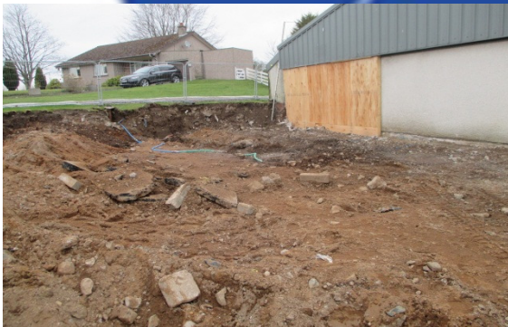
Old Lairage entrance cleared and ground prep ready for Gas Stunning Pit
