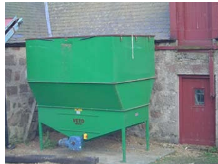
Hopper serving a 60kW boiler (image courtesy of Andrew Nicol of DWP Harvesting and Marketing)
